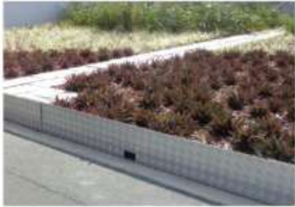
Provision of drainage outlet in greening to discharge excess water
