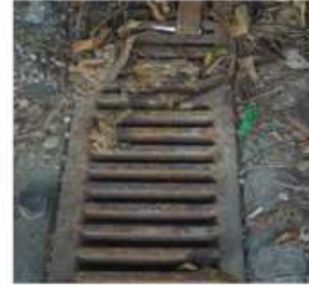
Improper maintenance of drainage system
