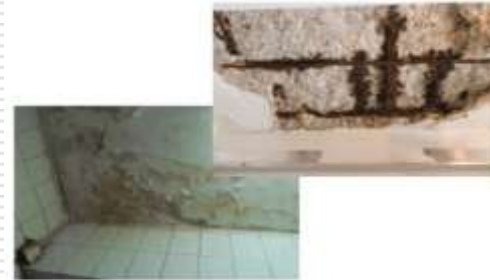
Inadequate or damaged waterproofing may result in water seepage and spalling of structural elements
